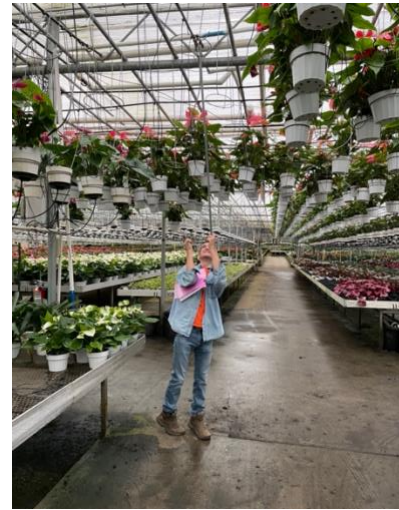
Above: I'm opening a valve to test a section of hanging irrigation.
